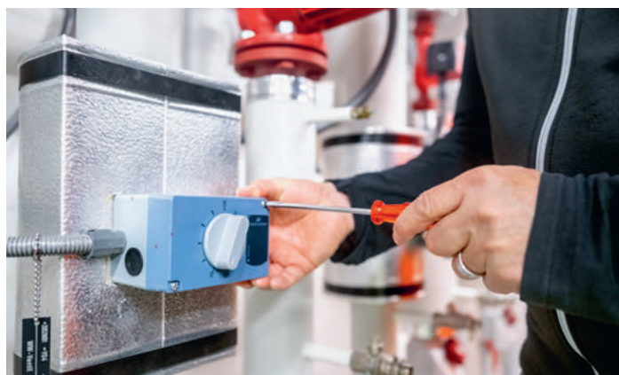
The laboratories at METAS rely on high-performance air-conditioning technology.
