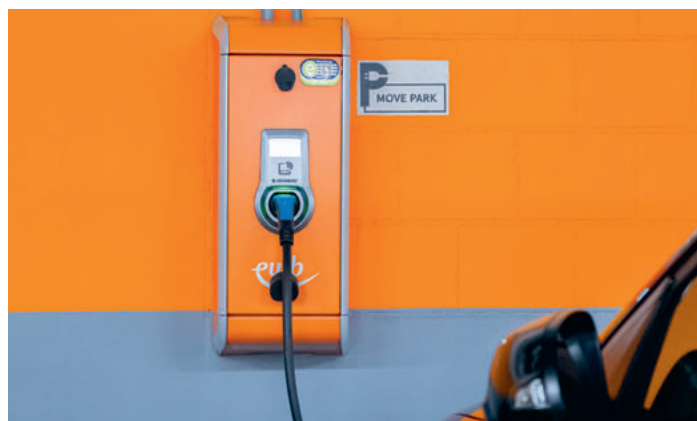
Electric charging stations: regulations for metrological requirements are being prepared.
